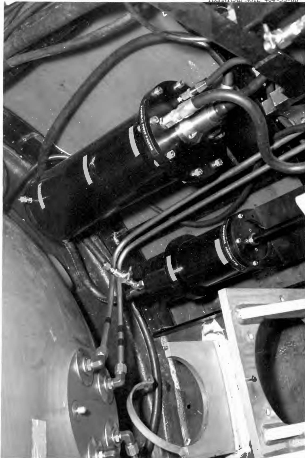
POWER PACKAGE (UPPER) FLUID MAKE-UP DEVICE (LOWER)
